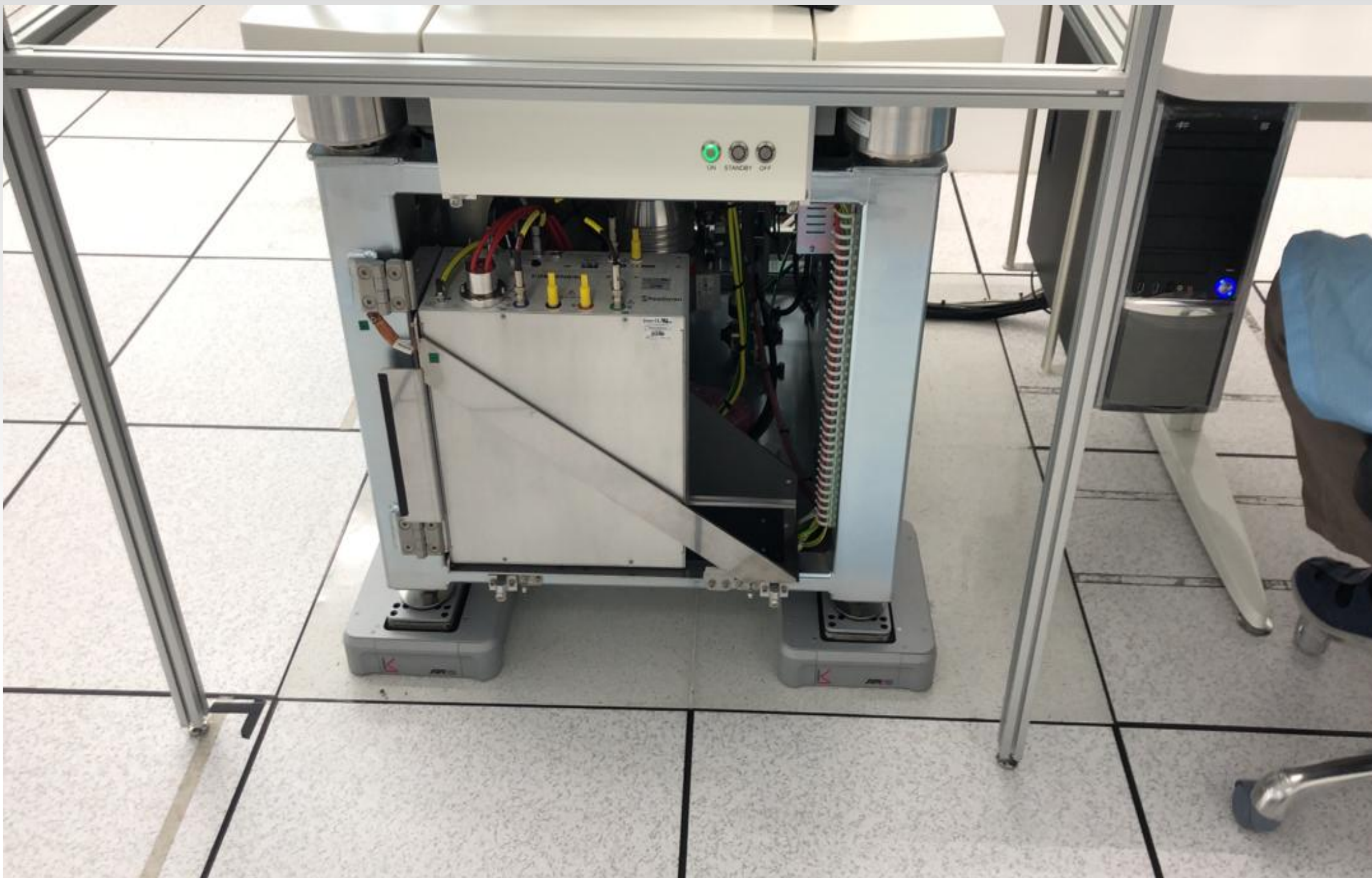
Zeiss Sigma SEM Installation on Raising Floor
