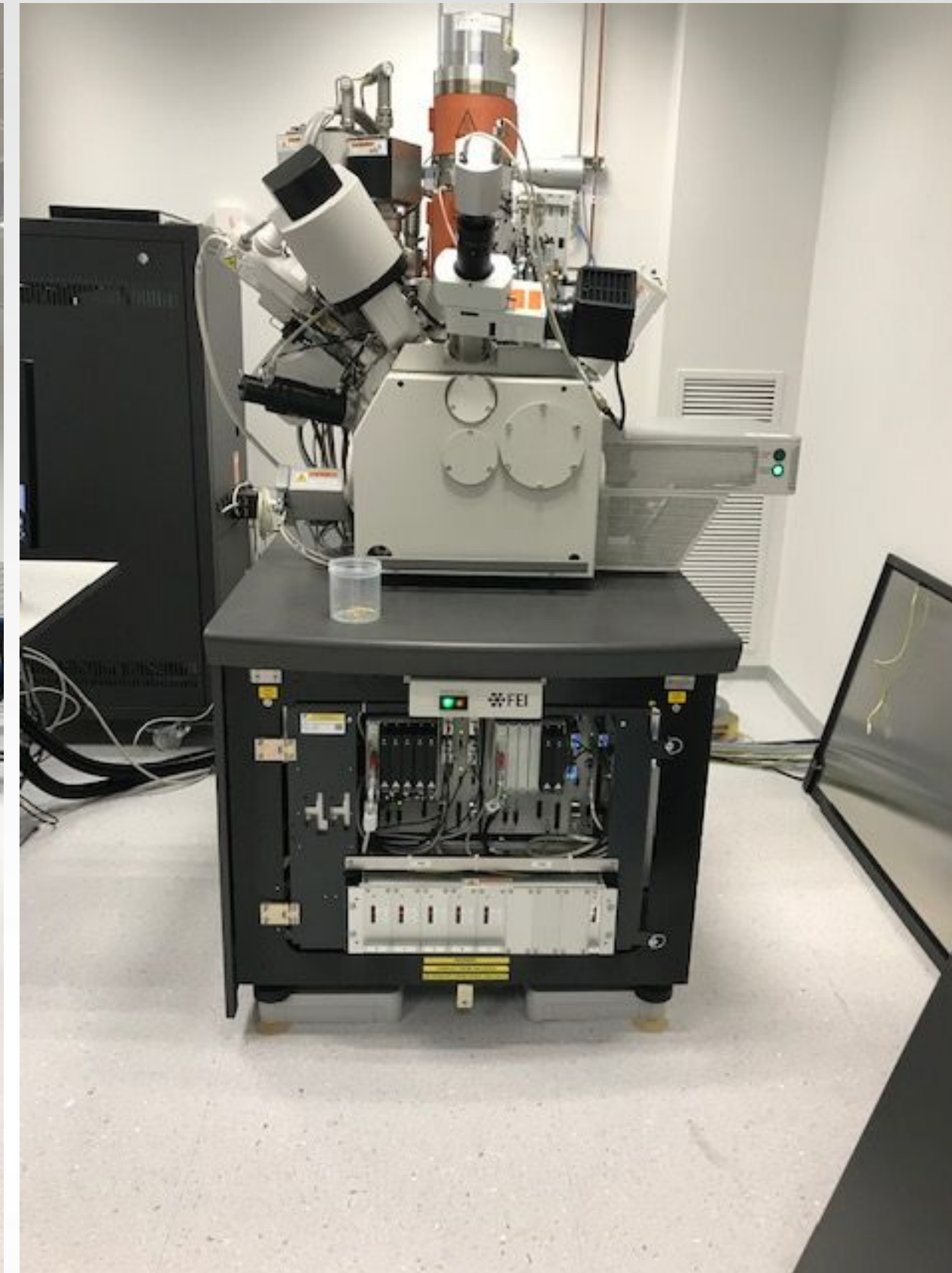
FEI Helios FIB Installed on 2nd Floor
